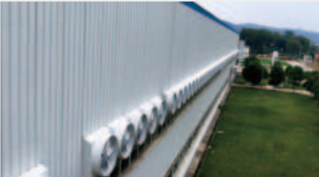
Home Appliance Factory
